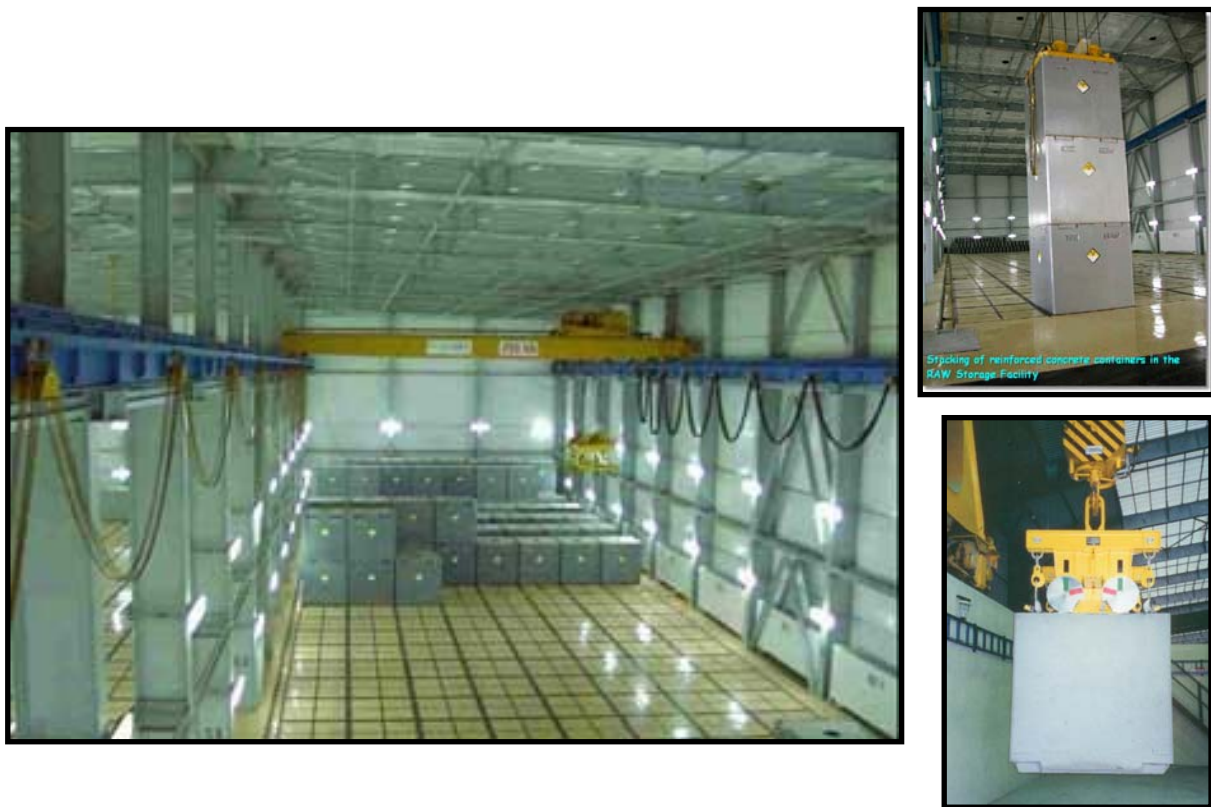
Figure 1.2-14 Reinforced concrete containers for low and intermediate level RAW
